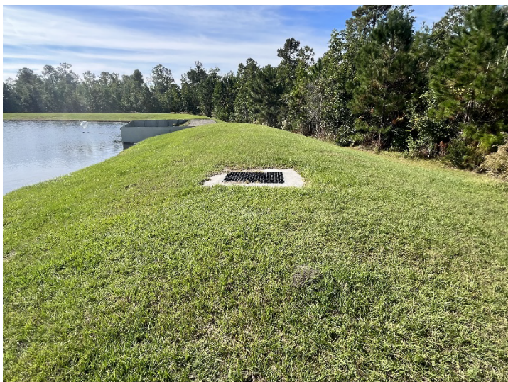
P-1 Control Structure
