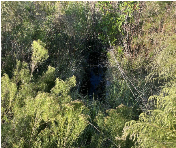
P-13A Outfall Mitered end section/riprap. (Overgrown Maintenance required)
