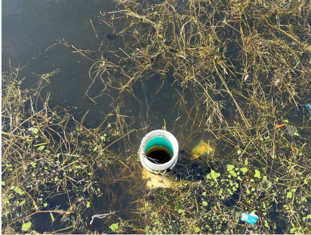
P-13C Replace Orifice Cap Maintenance Required
