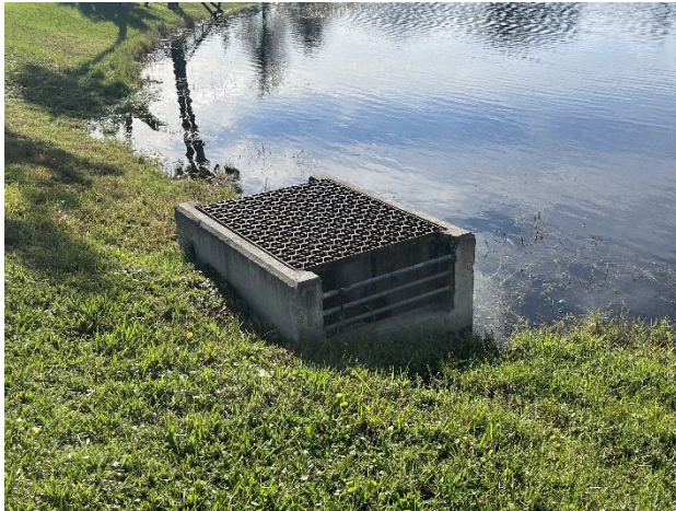
P-13C Control Structure
